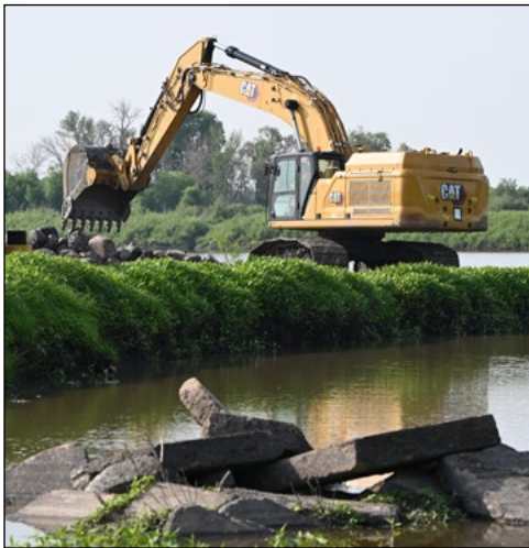
An excavator removes Drayton Dam, near Drayton, North Dakota, June 27. USACE St. Paul District photo by Patrick Moes
