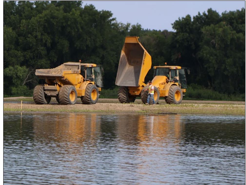
Construction continues at Pigs Eye Lake near St. Paul, Minnesota, Aug. 10. USACE St. Paul District photo by Elizabeth Stoeckmann
