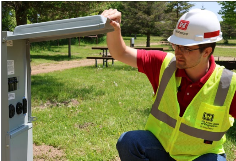
Mitchell Knegendorf, contracting officer representative, inspects an electrical panel at Eau Galle Recreation Area, near Spring Valley, Wisconsin, May 28. USACE St. Paul District photo by Dave Elmstrom
